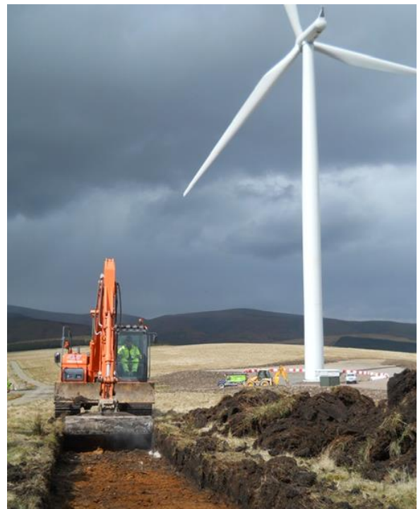
Controlled excavation of cable trench on the Clyde Wind Farm (© Headland Archaeology)
