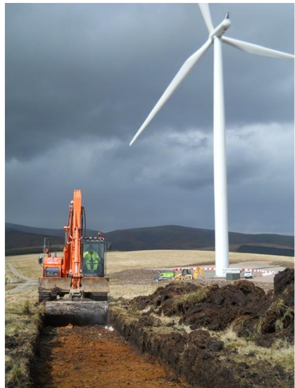
Controlled excavation of cable trench on the Clyde Wind Farm (© Headland Archaeology).
