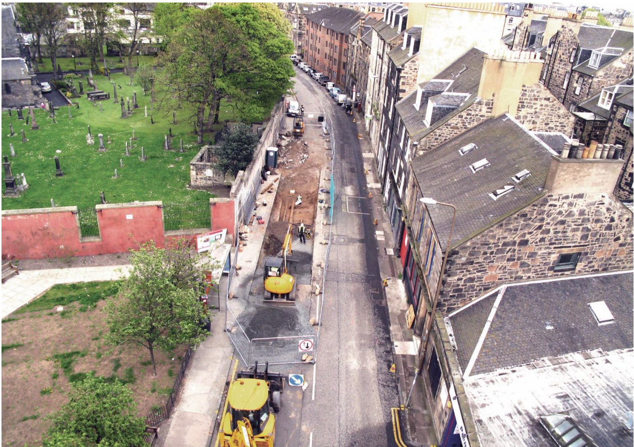
Aerial view of excavations in progress in Commercial Street, Leith, next to the Parish Church (© Headland Archaeology)
